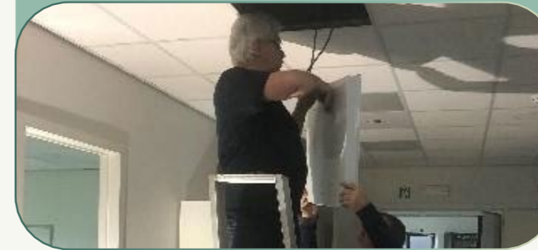
INSTALLATION D'ÉCLAIRAGE LED
