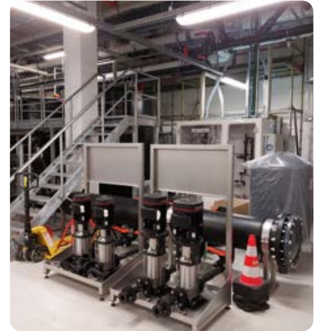
Water recovery plant (WRP)
